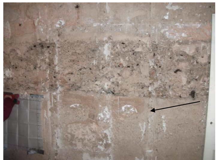
Figure 5. Tensile crack (arrowed) in concrete below centre deteriorated band - the crack did not extend into the centre band.
