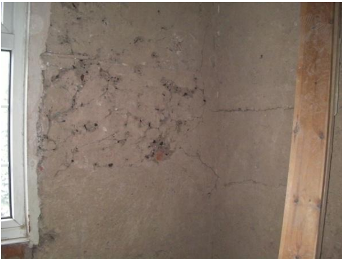
Figure 2. Internal cracking in concrete in upper wall
