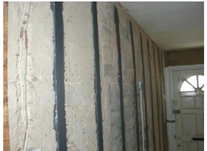
Figure 9. Carbon fibre strips glued in place with epoxy resin to provide additional strength to gable wall
