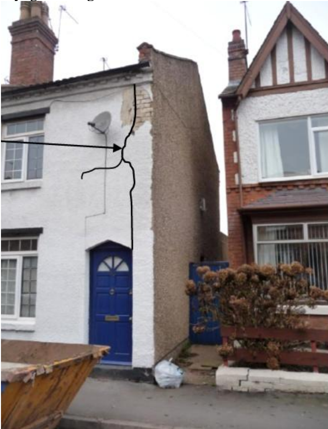
Figure 1. House showing crack (inked over) between gable wall and front elevation
