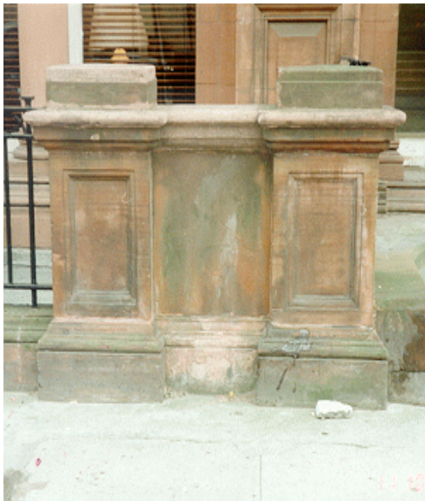
Damage of sandstone due to salt action
