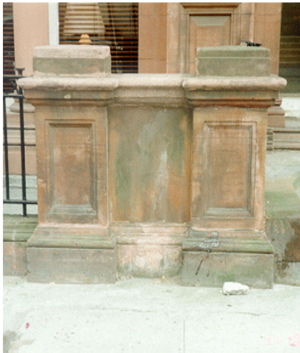
Damage of sandstone due to salt action
