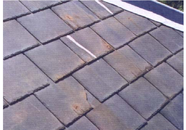
Deterioration of slate roof
