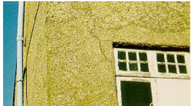
Cracking of render caused by deterioration of mundic concrete
