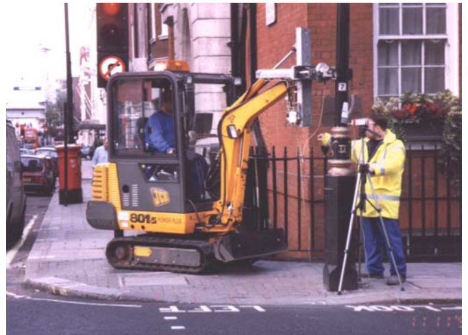
In situ load testing of a column carried out in conjunction with our partner, Roch Services Ltd
