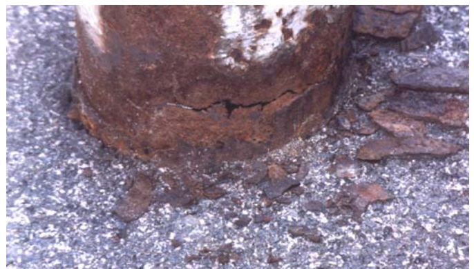
Poor condition of a column base. As can be seen from the surrounding debris, this crack was not revealed until the superficially sound surface was removed.
