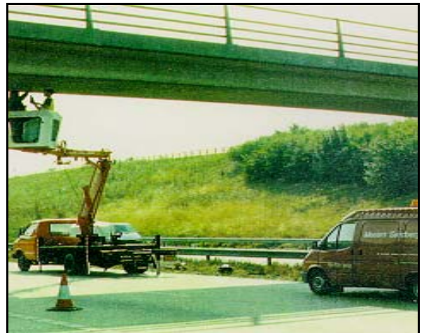
Testing under way on the deck soffit of a motorway overbridge structure
